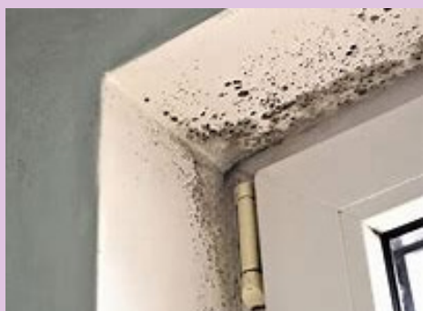
Typical mould growth from condensation.
