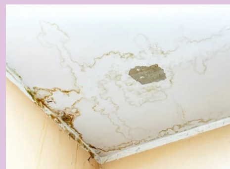
Signs of a leak or water ingress in your property (brown staining).
